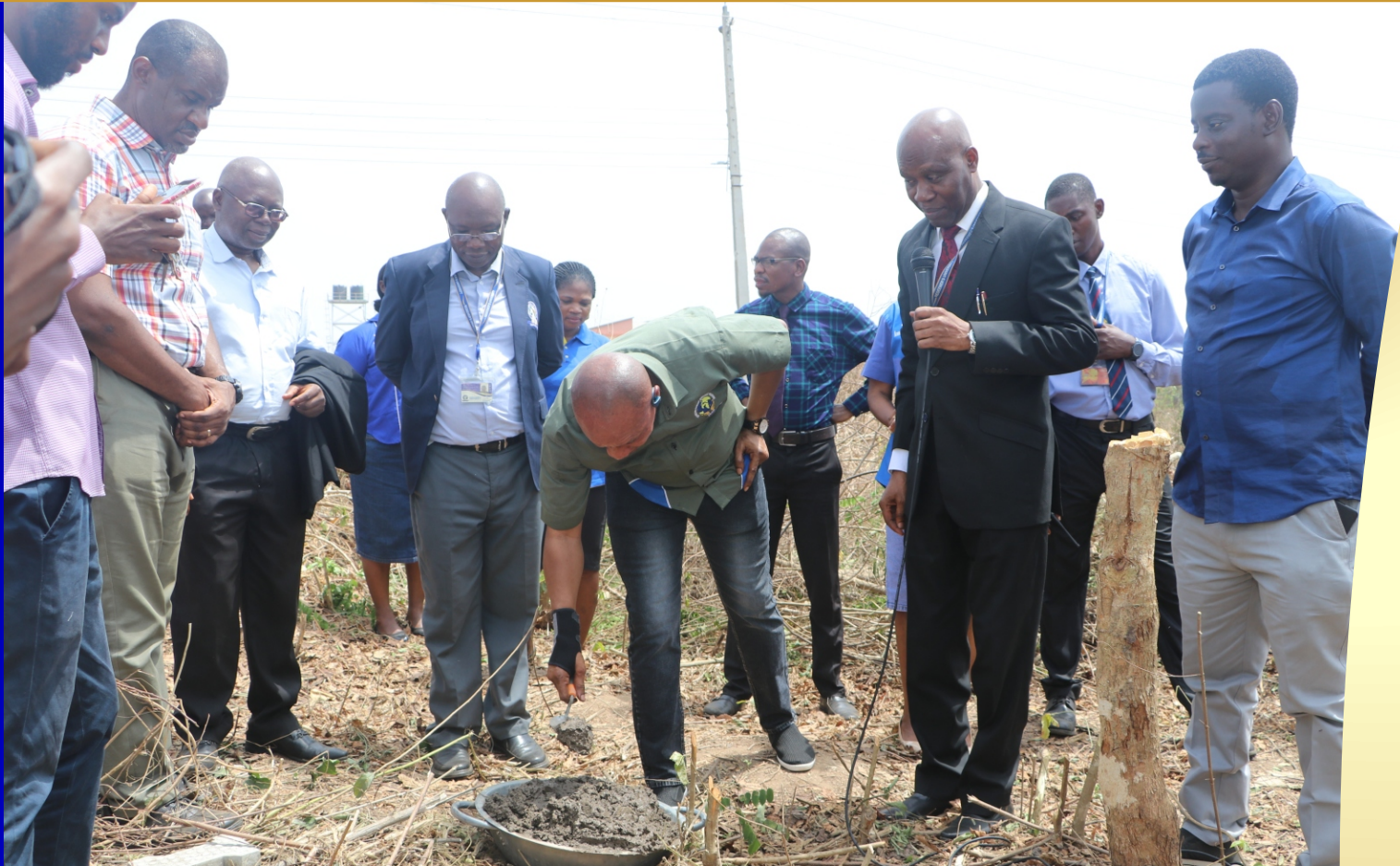
The foundation laying of 150-seater LH by the Chairman, SEAP, Pastor Olatunji Oladokun (JP), the Vice-Chancellor and other members of staff
